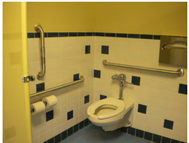
Typical handicap restroom stall
